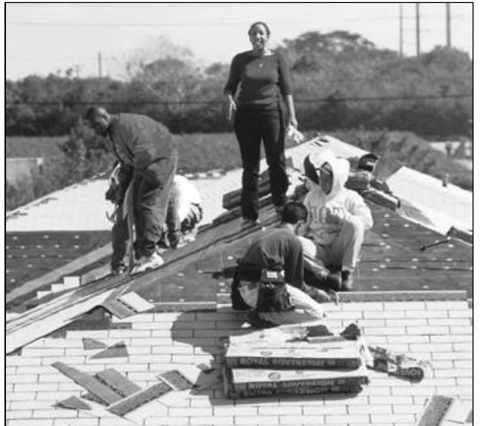
UM Law students and staff help renovate a home for Habitat for the Humanities, a H.O.P.E. outreach project.
